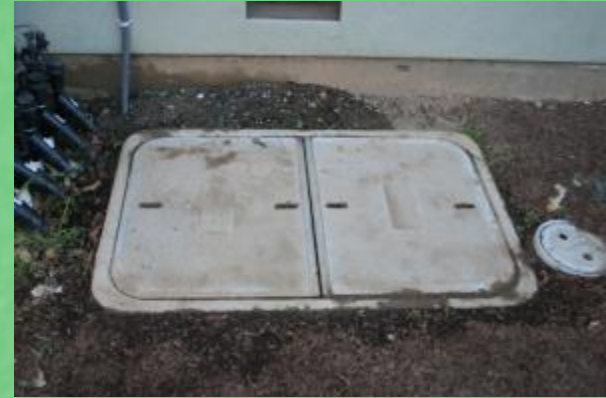
Surge tank in vault
