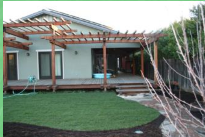
Lawn with subsurface drip tubing from Netafim, installed by EarthCare Landscaping, plumbing by Hal Branges
