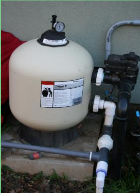
Sand filter from ReWater
